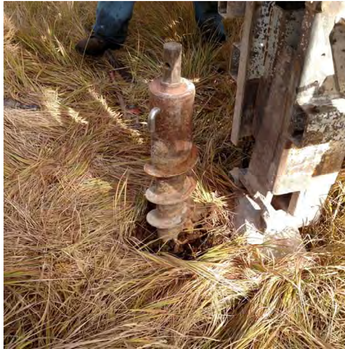
Well FB3 pre-installation looking north.
