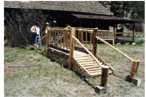
A bridge in Vallecitos, NM, built of small-diameter timber dipped in borate preservative, is one experimental product among others.
